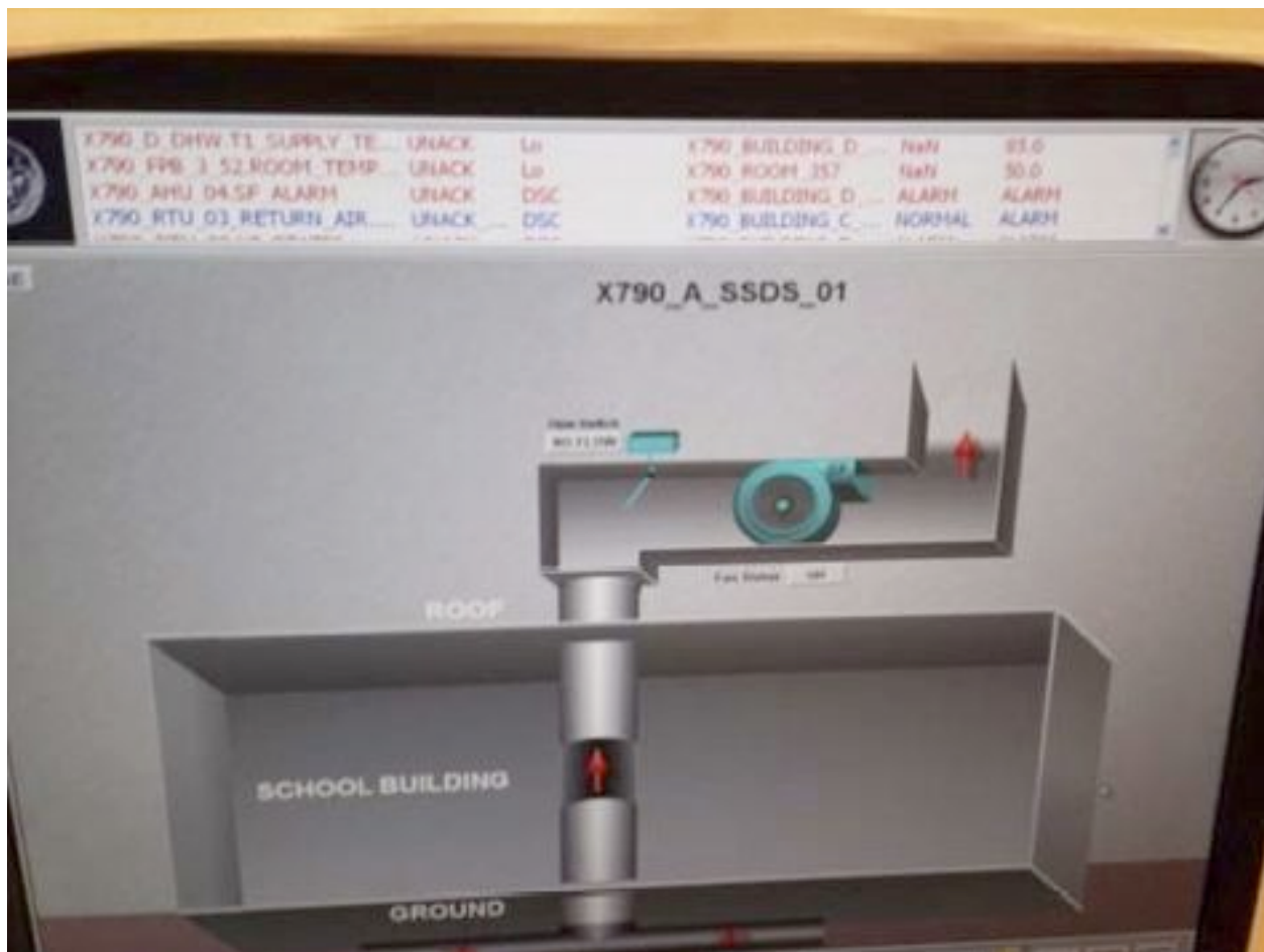
Building Management System for monitoring mitigation fan at a Bronx, New York school
