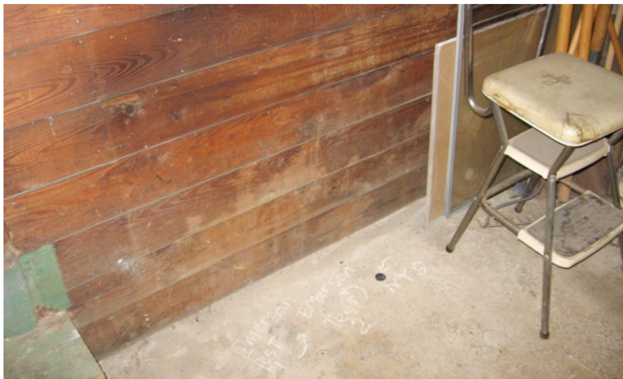
Plugged sampling hole in Ithaca, New York basement
