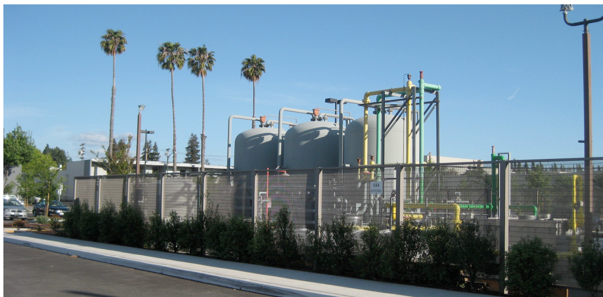
Carbon adsorption system for groundwater treatment
